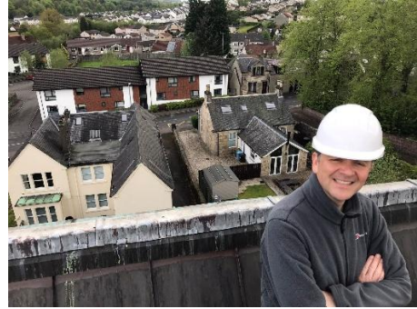
Fr Deeley inspecting repair works to the roof of St Patrick's May 2023
